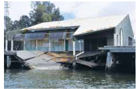
Collapsed wharf at the western end of North Wharf.
