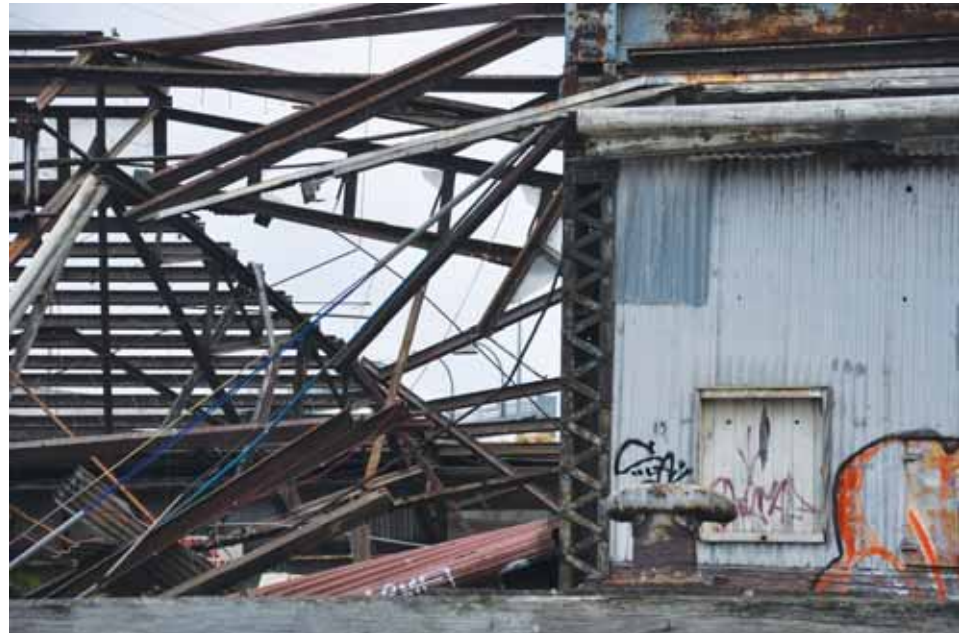
The damage at Sheds 20 and 21.
