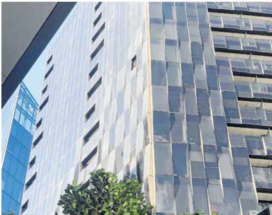
A window from the side of a Docklands Drive building last month popped out due to high winds.
