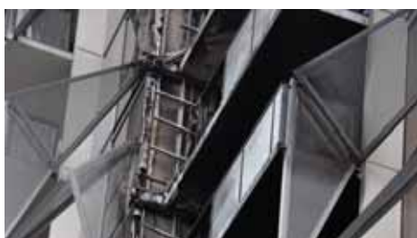
Damage to the building’s exterior caused by the fire.
