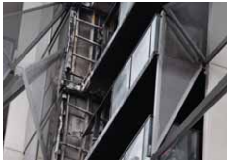
The cladding investigation was launched following the Lacrosse fire.
