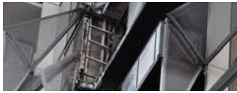
Damage to a balcony following the Lacrosse fire.
